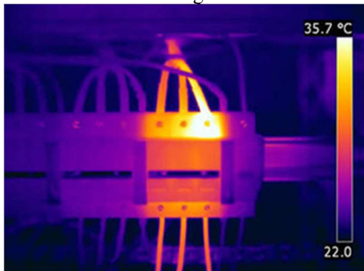
Fig. 1. Termographing an electrical panel [3]
