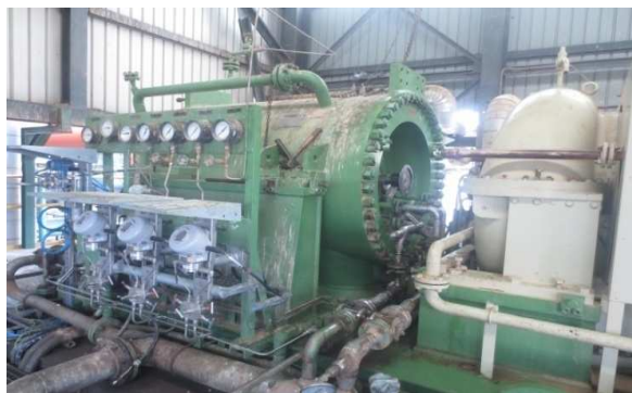
Fig.2. Compressor installation studied
