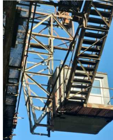
Fig.2. The real operator cabin
