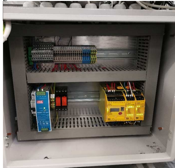
Fig. 2. Electrical panel for controlling the auxiliary safety system in applications with collaborative robots
