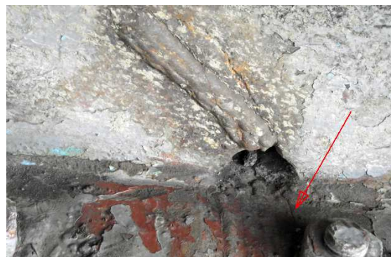
Fig.1. Crack at the rotating platform after a repair
