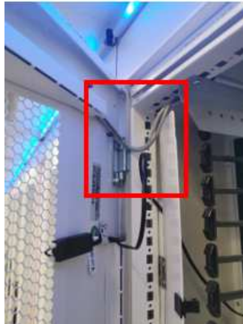
Fig. 4. High Break Risk Cable Assembly
