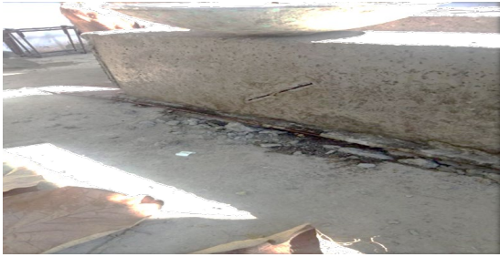
Fig. 8: Preformed crack beam
