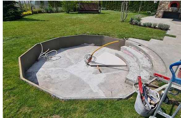
Fig.2. Another company's solution that offers a polygon shape, as round cannot be achieved by their technology
