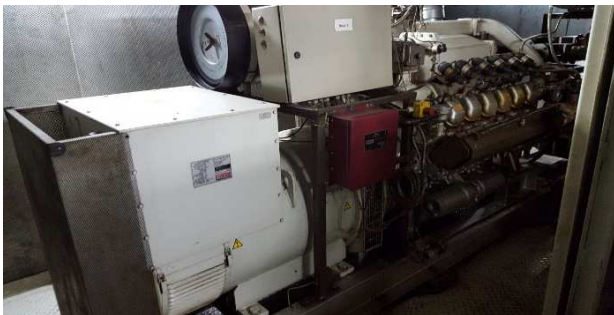
Fig. 2. Medium size Cogeneration Group
