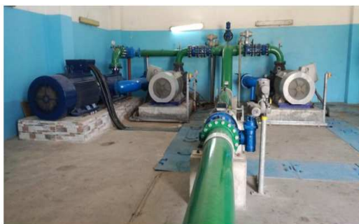
Fig. 2. View of SP1 station and Moto pump units
